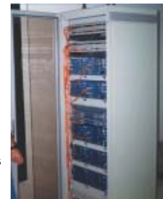
EOTec 6000 Modems installed in Control Room rack system
